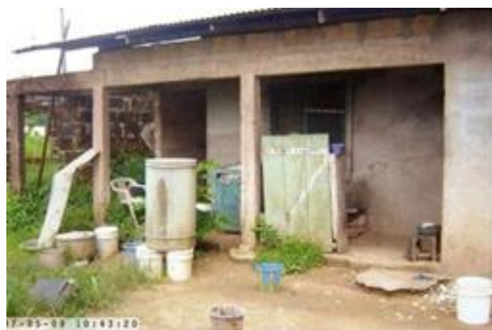
Figure 14. Chief Benjamin's one-story building at Okoroba village with a temporary roof covering over a part of it.
